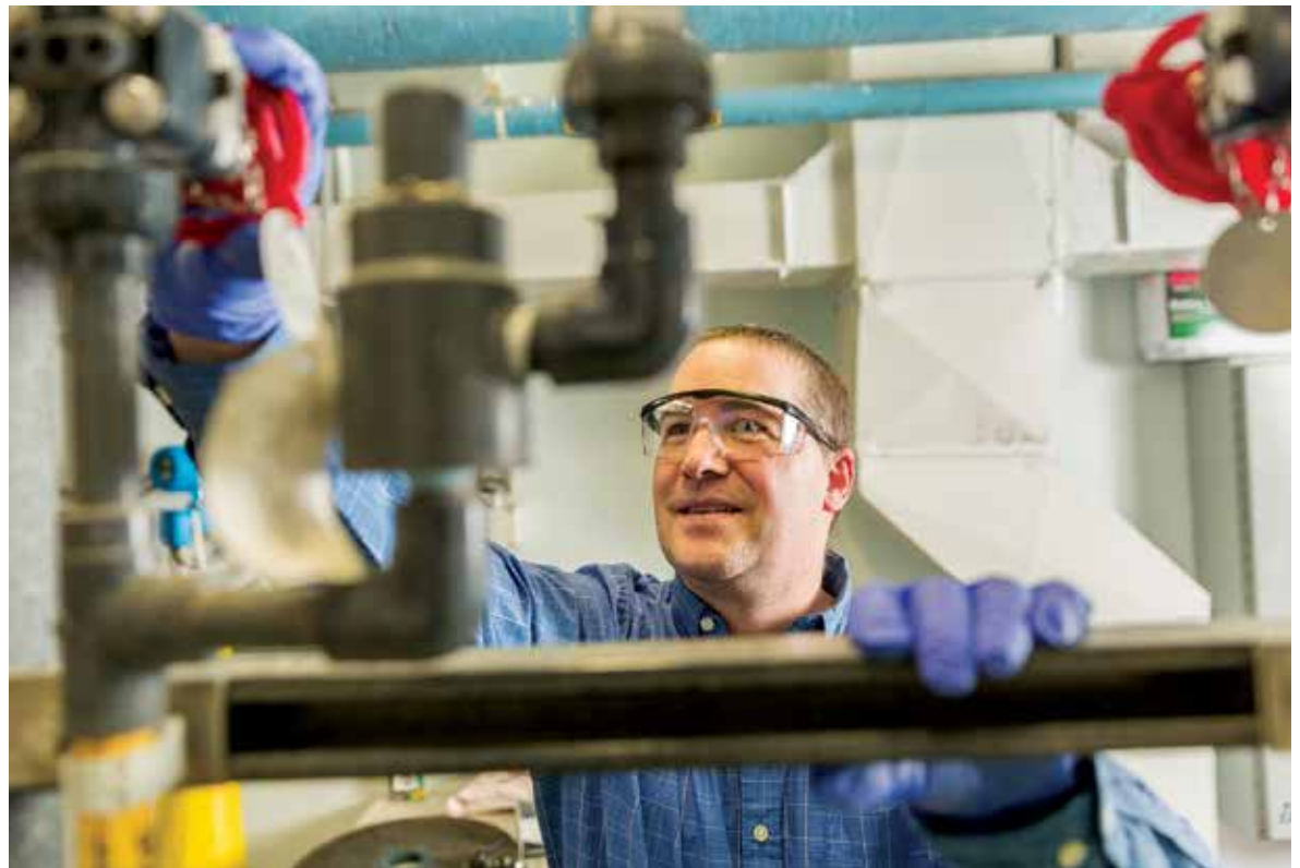
Timothy King tests for chlorine residual (upper photo) while Dan Driscoll swaps a chlorine pump as part of a regular rotation.
