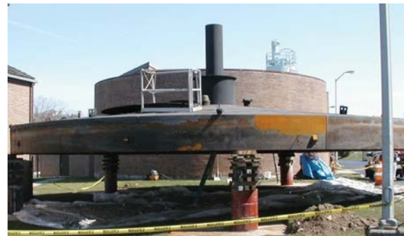
Expertise for all anaerobic digestion systems
