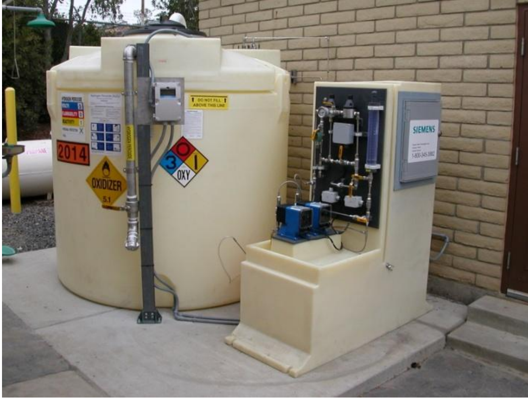
Figure 4 – Polyethylene Advanced Dosing System
